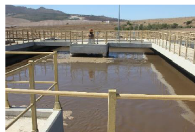
Reactor: Anoxic zone with two mixers
