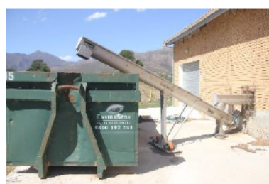
Dry sludge conveyor system (Huber)
