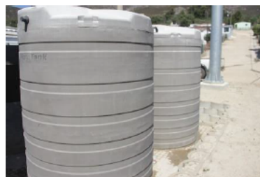
Three Aeration Tanks
