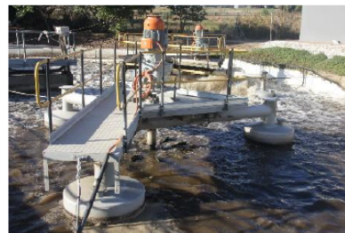
Reactor: Floating aerators
