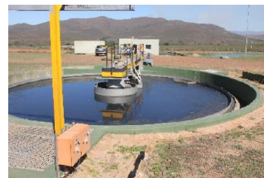
Secondary Settling Tank
