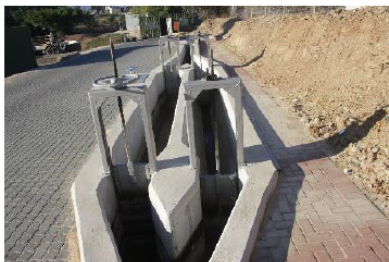
Inlet works with two grit channels
