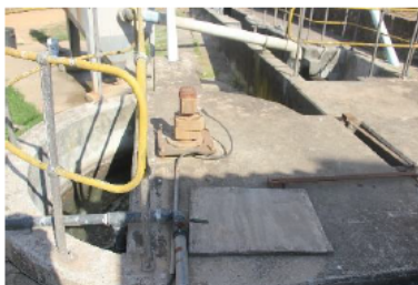
Inlet structure: Two vortex degritters
