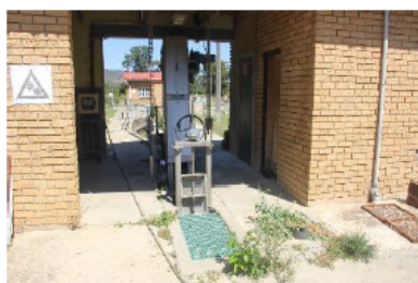
Inlet Structure with mechanical screen
