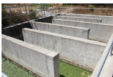
Chlorine contact channel
