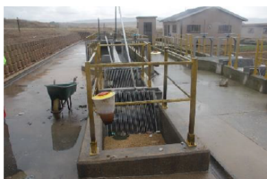
New Inlet works with 2 hand raked screens
