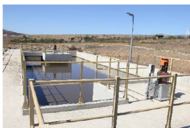
Reactor: Anaerobic zone with two mixers
