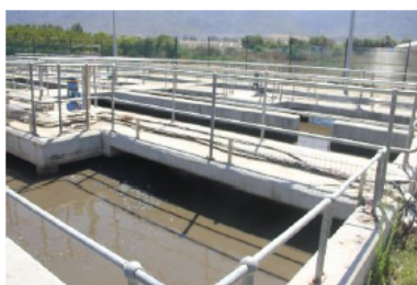
Reactor: Anaerobic Zone
