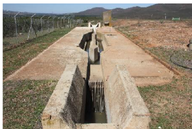
Inlet Structure with hand raked screen
