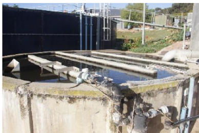
Chlorine contact tank
