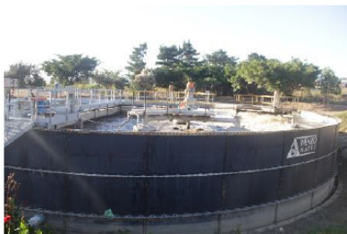
Sequencing Batch Reactor, with floating aerators
