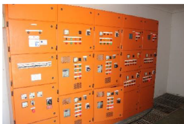
MCC for plant
