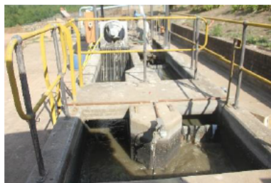
Inlet structure with mechanical screens
