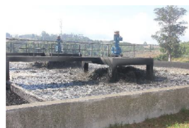
Reactor: Aeration zone
