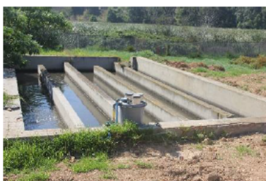
Chlorine contact channel
