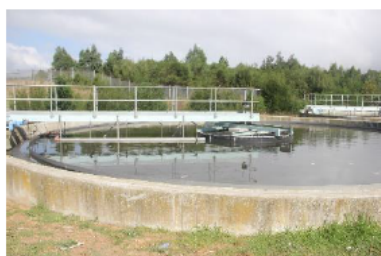
Secondary Settling Tank No.5
