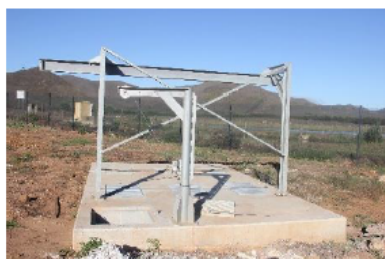
Raw wastewater PS
