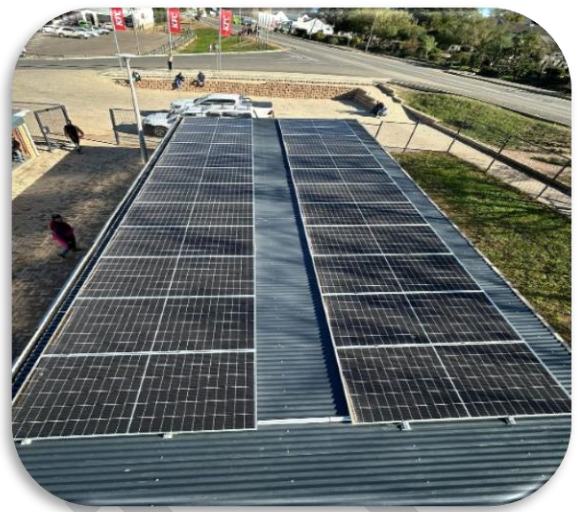
Solar Panels installed at Villiersdorp Trading Market as part of the AESP Pilot
